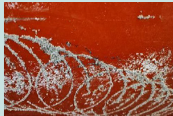
Vertical sides of a tanker coated with an FRC. Barnacles attached to mechanical damage areas. In service period: Unknown.
